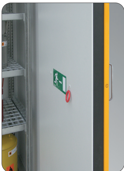
emergency opening device
